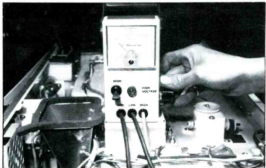
Figure 2. A defective magnetron may be detected by taking voltage and current measurements with the microwave oven Magnameter.
